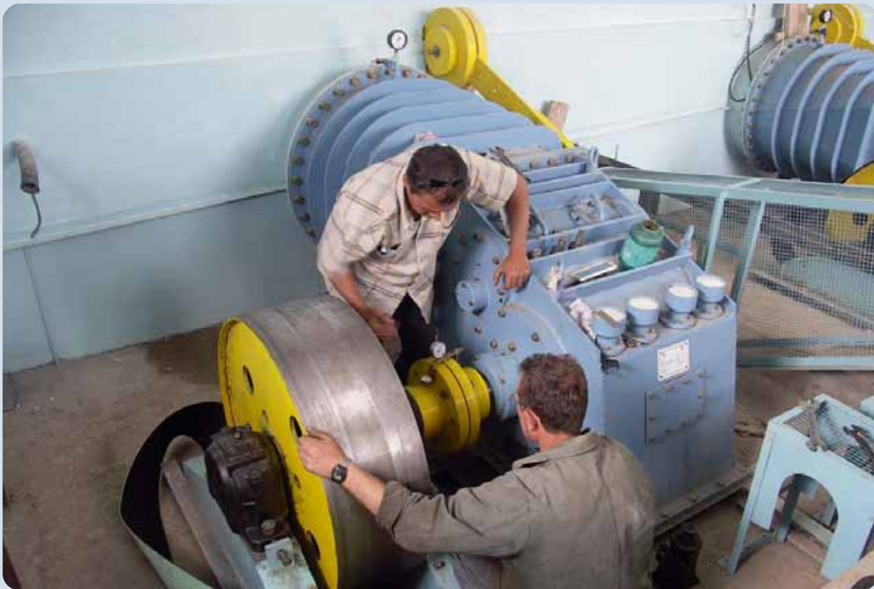
Installation of an entec T15-500 turbine with flat belt in Kirgistan
