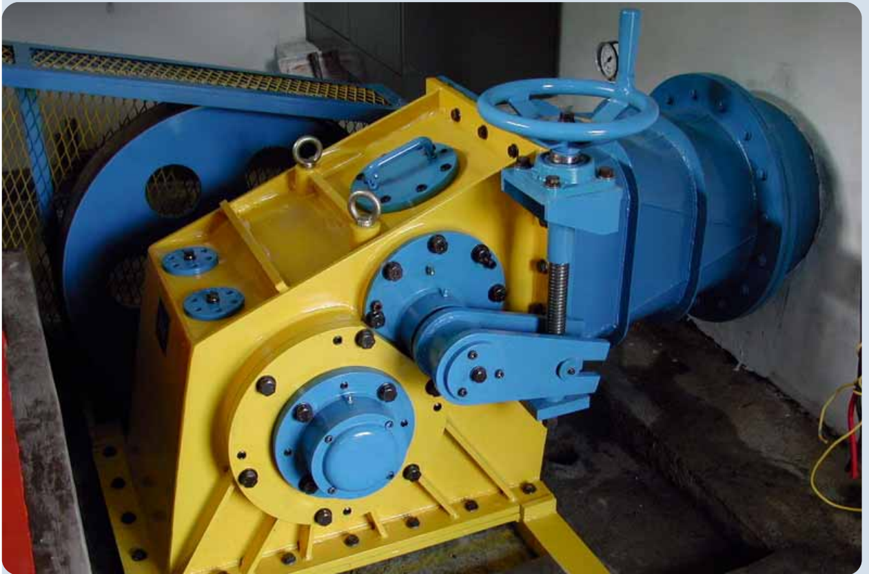
Entec T15-300 turbine, coupling on turbine shaft; produced and installed in Indonesia
